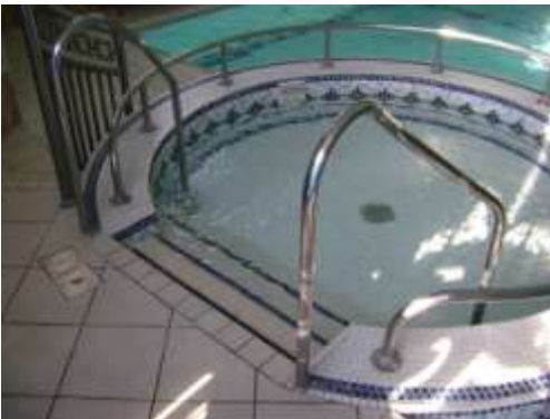
There are 4 x steps into the children's pool with handrails to both sides.
